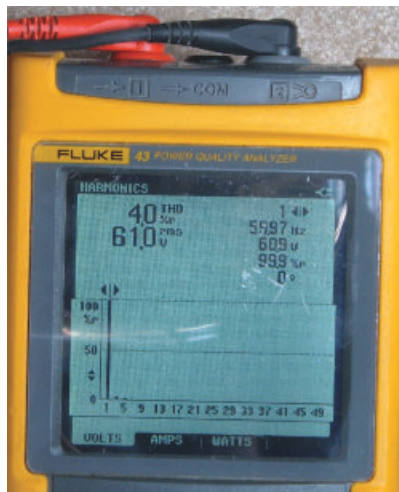
Photo 2 Showing clean AC flowing in the separately derived power system for the author's acoustic lab.
