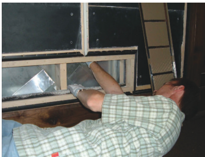
Photo 1 The author installing a constrained-layer damping treatment to an existing noisy HVAC duct.
